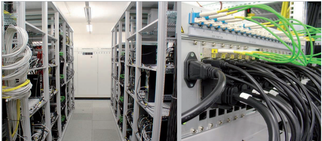
Patch panels in the system room
