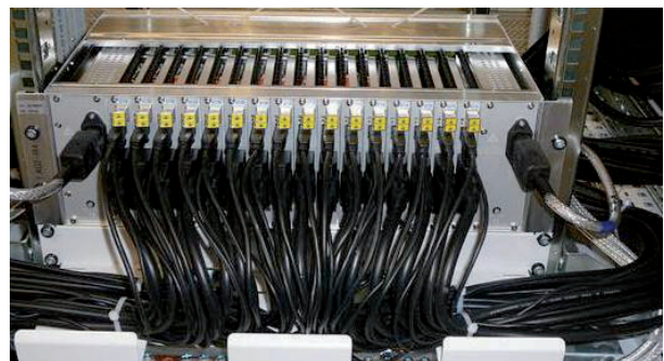
The patch panel in the system room
