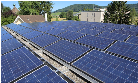
Rooftop solar panels at HQ
